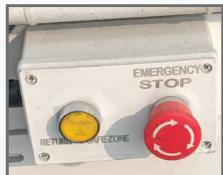
Emergency Stop in Bucket
